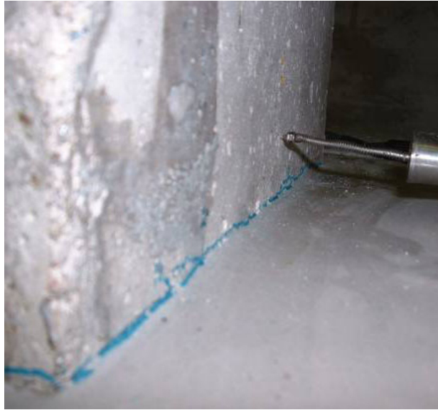
b.) West face initial cracking
