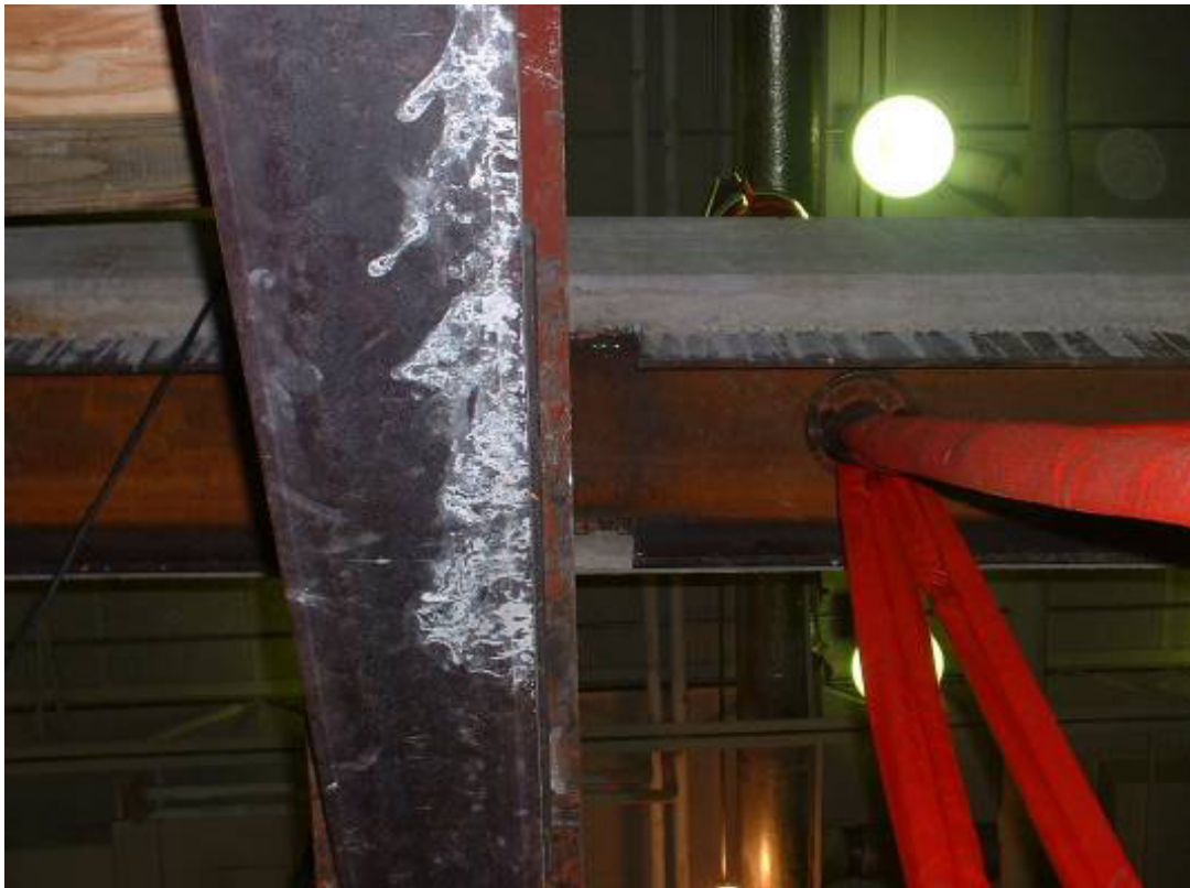
c.) Load beam impinging on load frame
