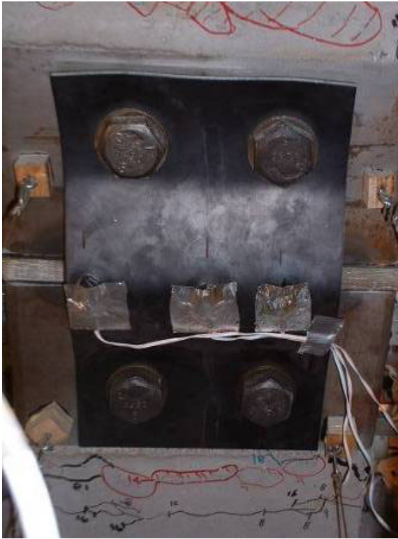
a.) West face damage and fuse plate buckling
