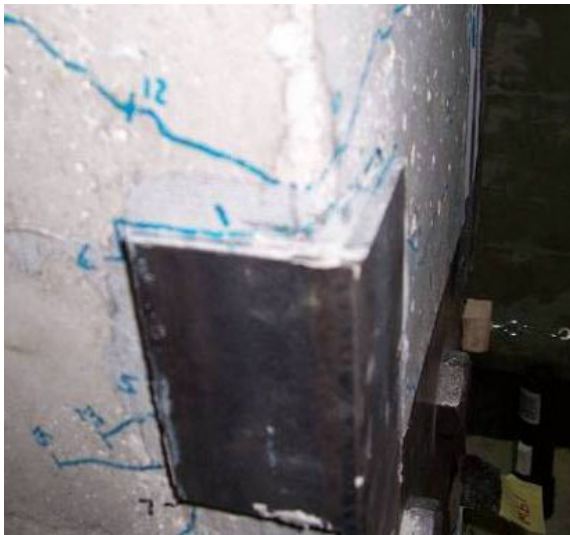
a.) Cracks forming around southeast retrofit angle
