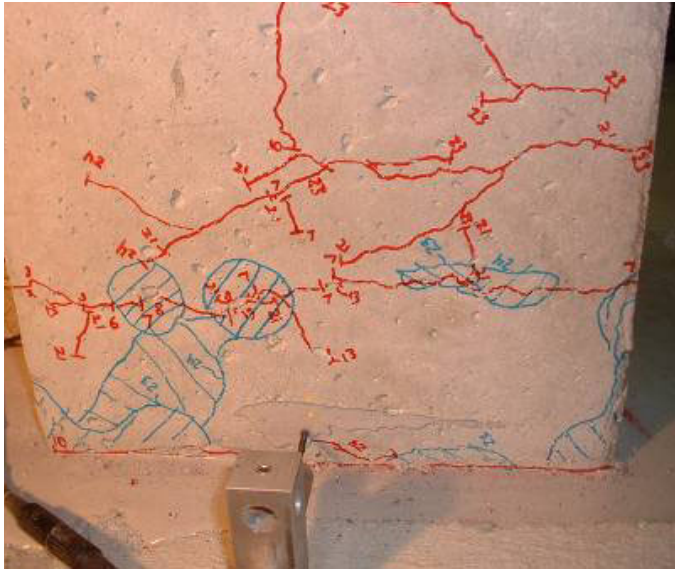
a.) East face damage
