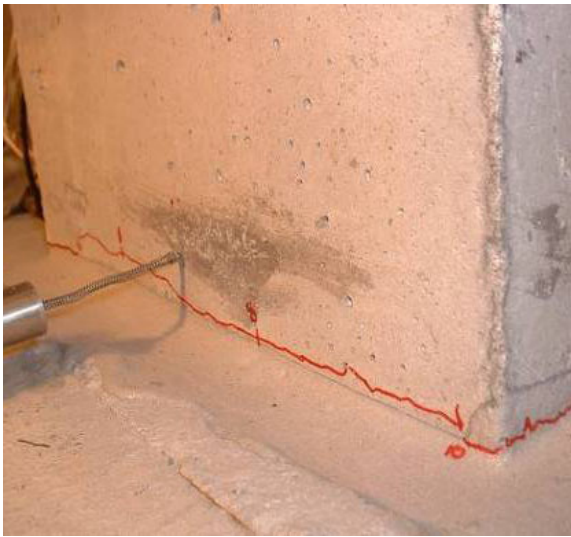
a.) East face initial cracking
