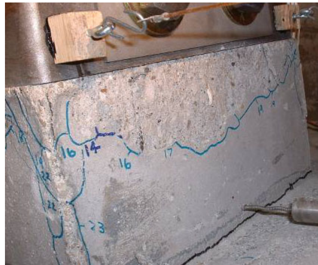
b.) Lower segment west face spalling
