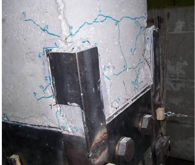
b.) Upper segment damage and retrofit failure
