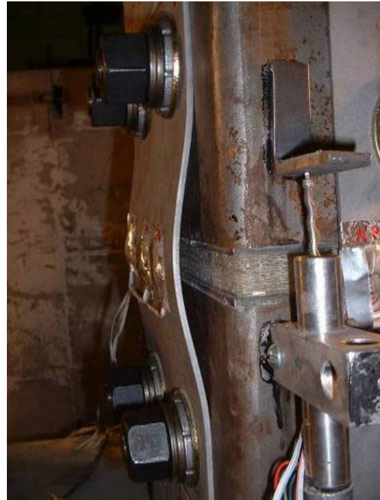
b.) East fuse plate buckling
