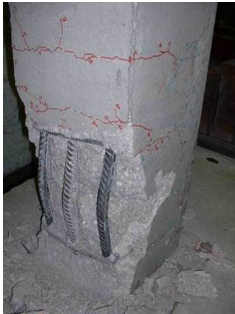
c.) Final damage to east face
