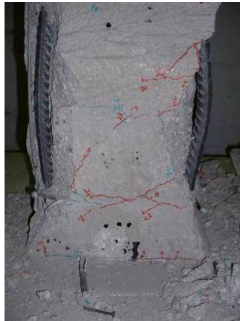
d.) Final damage to south face
