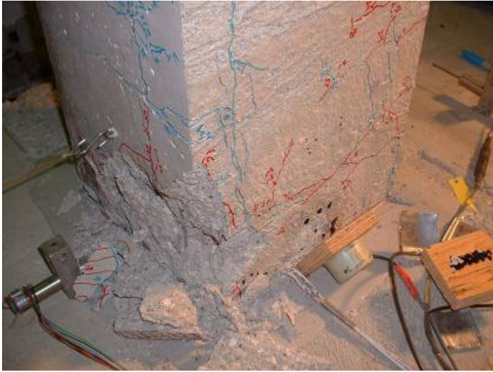
a.) Severe spalling of southwest corner
