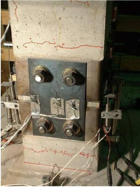
a.) Cracking around column joint
