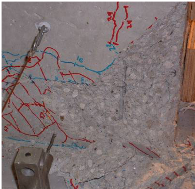
a.) Southwest corner damage
