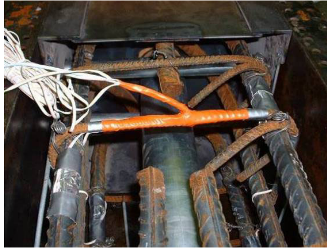
Figure 47. Photograph of Column 4 collar region congestion.
