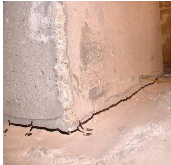
b.) West face initial cracking
