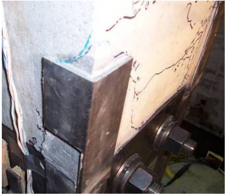
b.) Incipient cracking at southeast retrofit angle
