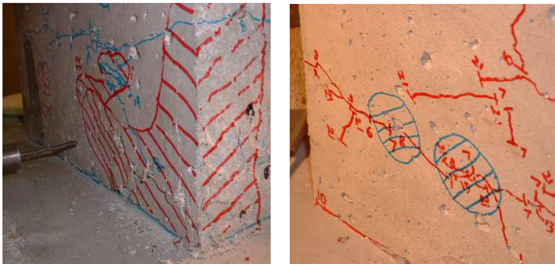
a.) Southwest corner compression damage
