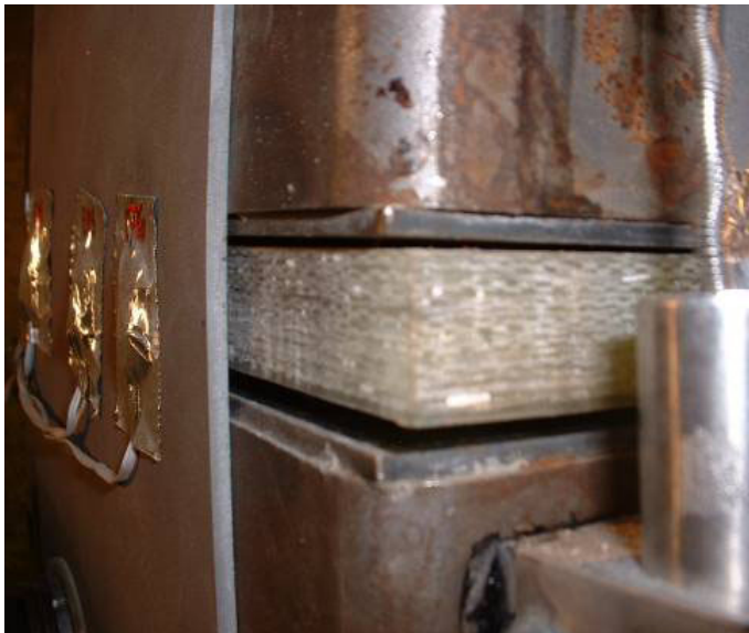
c.) Northwest corner joint opening
