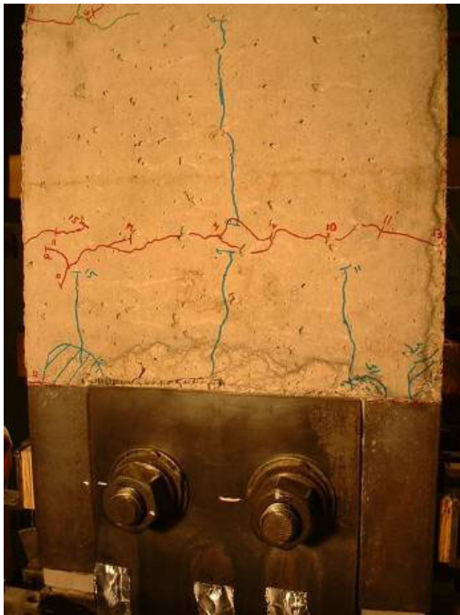
c.) East face cracking above top collar
