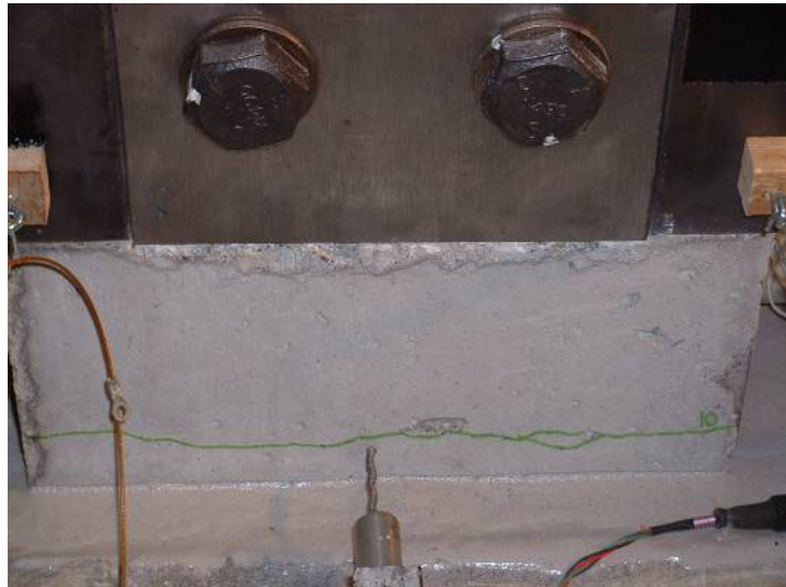
b.) West base initial cracking
