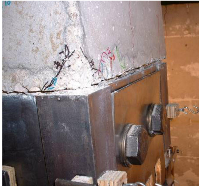
b.) West collar/column interface final crack width
