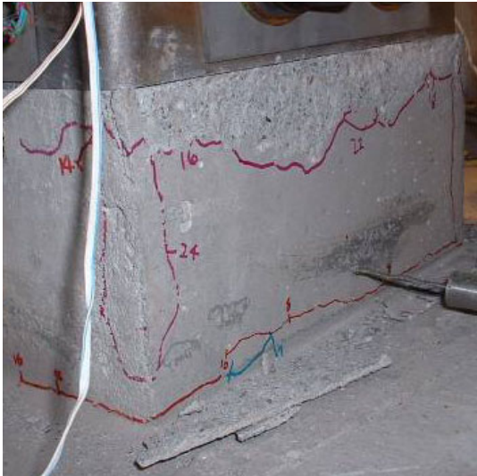
a.) Lower segment east face spalling
