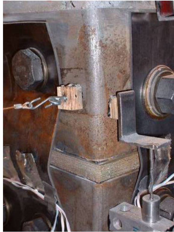
b.) Southwest corner fuse plate buckling
