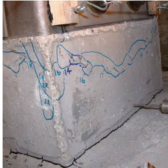
b.) Lower segment west face compression damage
