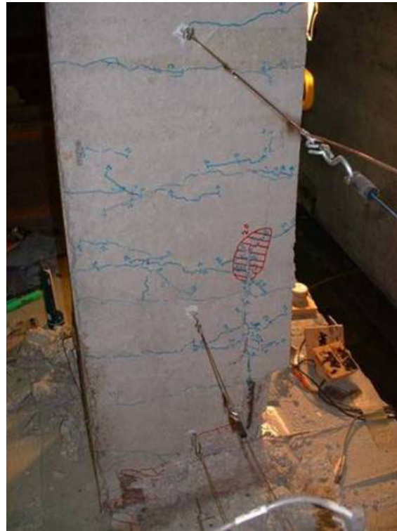
d.) West face damage
