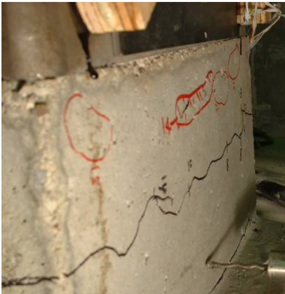
a.) West face compression damage and cracking at base
